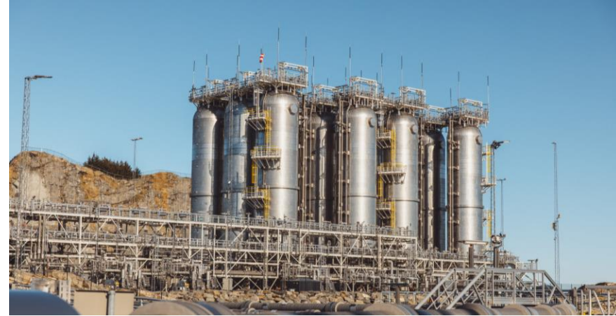
Above Northern Light LCO 2 terminal with vertical tanks at Øygarden, Norway ( https://norlights.com/ )
